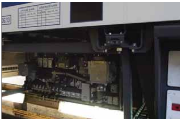
2. ábra: Fékonténer a BRT698- as fékpanellel Abb. 2: Bremscontainer mit Bremspaneel BRT698 Fig 2. Brake container with type BRT698 brake panel.
